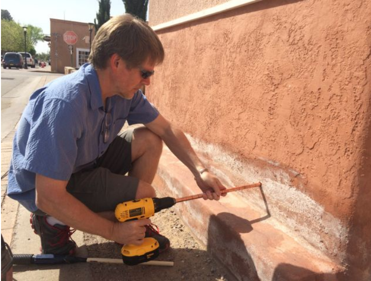
Figure 2. Core samples are taken at one-inch increments using a specially designed coring tool, with care to avoid sample cross-contamination.
